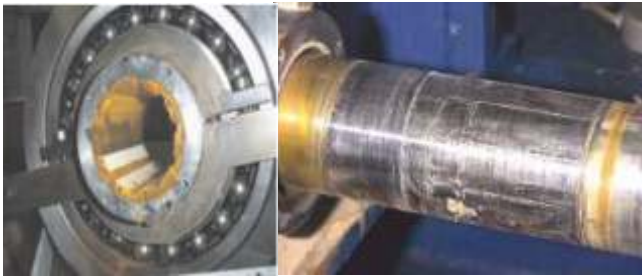
Elastomeric bearing wiped & Shaft Condition
