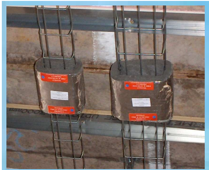
Cable Basket Fire Sleeves Installed On-Site
